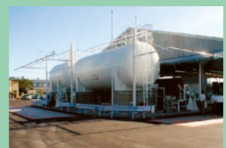
LP gas filling station
