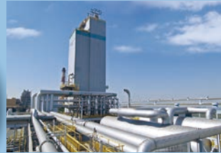
Gas supply pipelines
